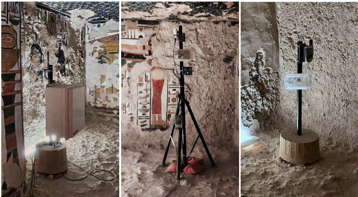
>> Figure_4.2.14. Equipment for the tomb's microclimate monitoring system Photo // François Olivier, Tatiana Nikolaychuk
